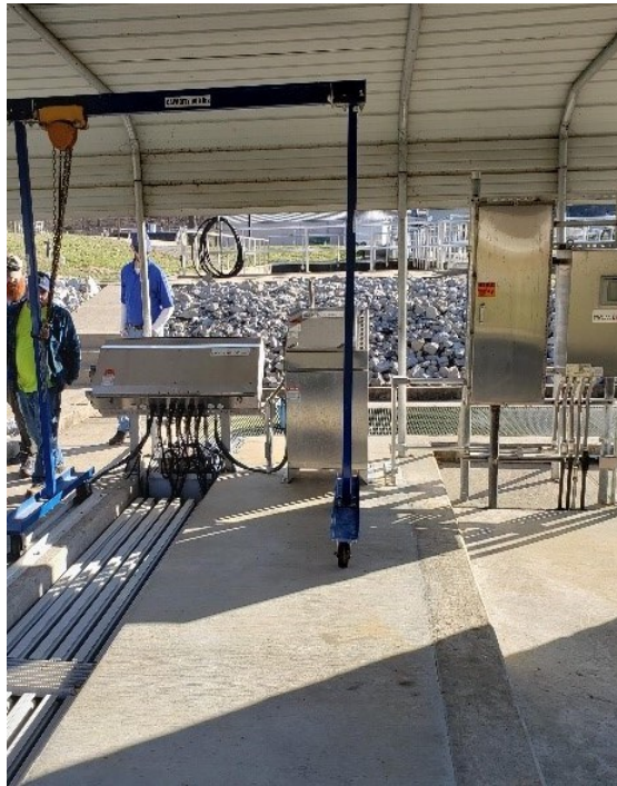
Above: Radcliff Wastewater Plant's headworks.
